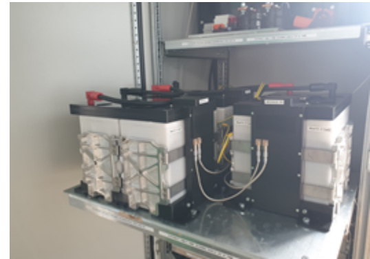
3 modules of the big battery pack on a cabinet sliding shelf
