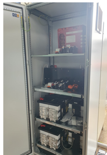
Battery Pack Cabinet with inside 6 modules of NiZn cells, DC-DC converter, power Unit-BMS and connector blocks (side DCDC and inverter) work.
