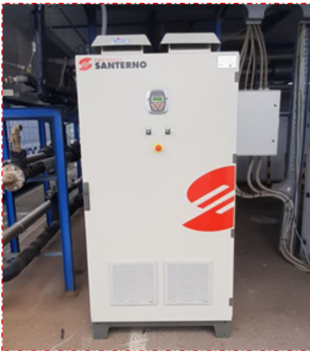
The purchased Inverter Santerno for the connection of the battery pack to the Savona campus smart grid
